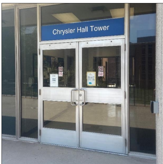
Additional entrance located on the south side of the building - ground level with no actuator.
