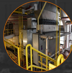
Sustainable hybrid chiller plant
