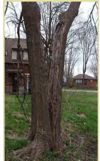
Photograph 7. This split trunk on University property presents a Severe-Risk to the community and should be removed as soon as possible.
