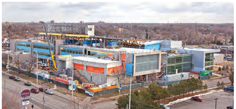
This photo of the Centre for Engineering Innovation was taken from the tower of the Odette Business School in January 2012. With most of the concrete work now completed, the tall central crane which had been a fixture on the horizon for nearly two years has been removed.
